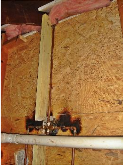
Cut wall stud not properly drilled or supported. Shower valve not properly secured to the framing to prevent movement/ potential leakage. Uninsulated wall against the shower. Water piping in an unconditioned spaces; potential freeze issue. Excessive scorching of the adjacent wall materials from an adequate soldering procedures.
