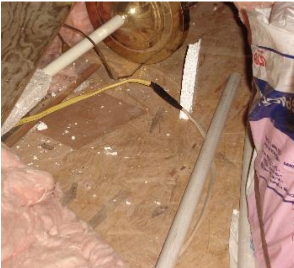
Visible spliced wire outside of a junction box in the attic.
