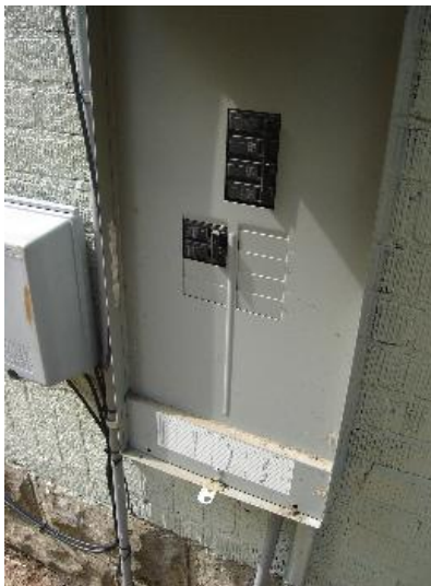
Main electric service panel not labeled as required.
