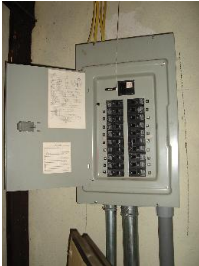
Main electric subpanel not properly labeled. Romex wiring installed on the outside of the finished wall system.
