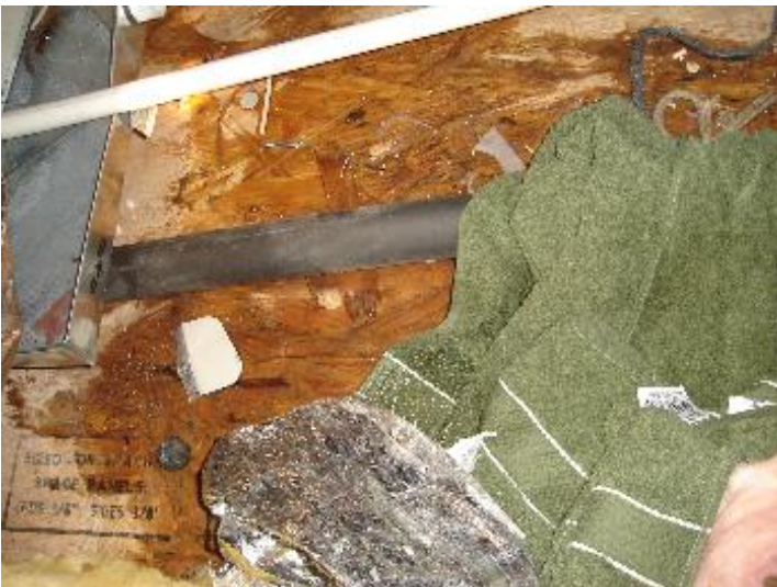
Water damage on attic flooring. A towel was present (apparently the leak was known earlier).
