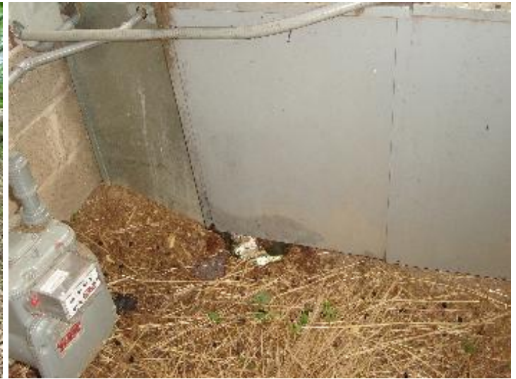
Leaking condensate/drain pan/frozen coil.
