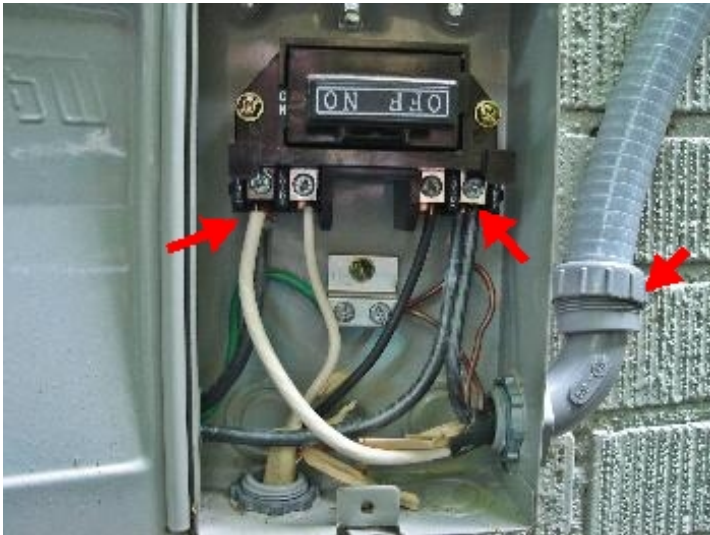
Double tapped electrical supply at the new outdoor HVAC unit. Liquid tight connector not properly installed; cross threaded.
