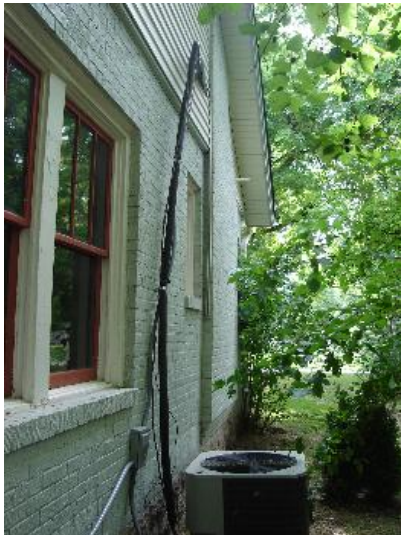
Improperly supported refrigeration line sets. Improper termination of the condensate drain line overhead.
