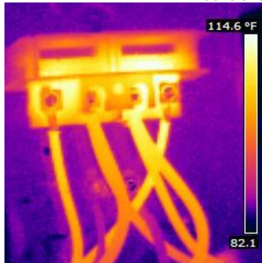
Overheated condition of the first floor HVAC disconnect. Disconnect components are overheated as well as double tapped electrical wiring. There is no overload protection for this wiring size observable. Double tapping creates an overloaded condition which is apparent in this case.
