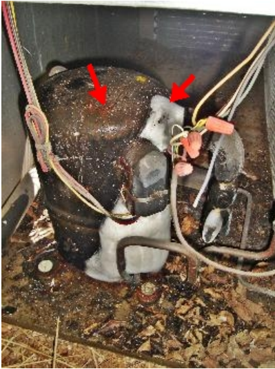
Frozen first floor air-conditioning compressor. Restricted airflow at coil. Low refrigeration pressures. Equipment requires dismantling/inspection and servicing. Rusted compressor head indicates an ongoing past occurrence of this condition. Evaporator coil is likely restricted.
