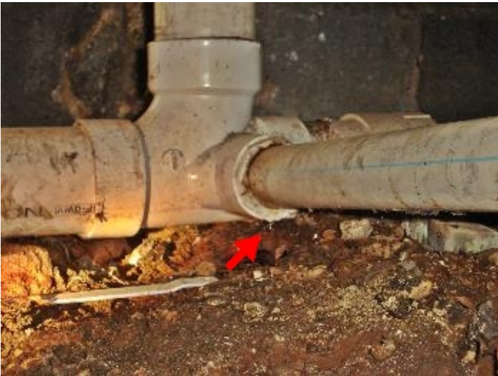
Waste drain leakage observed
