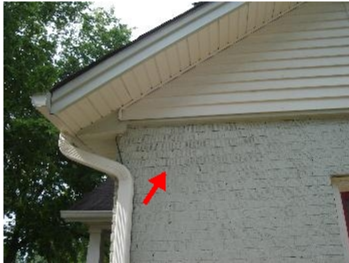
Minor step crack.
