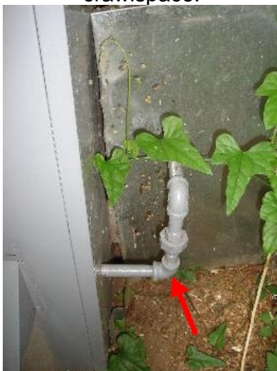
No drip leg on gas piping.
