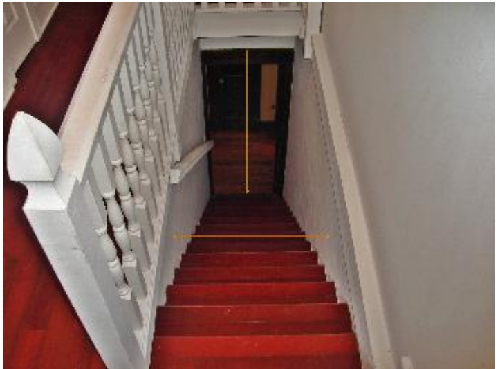
Stair system is less than 3 feet wide. Staircase header less than 6'8" high.
