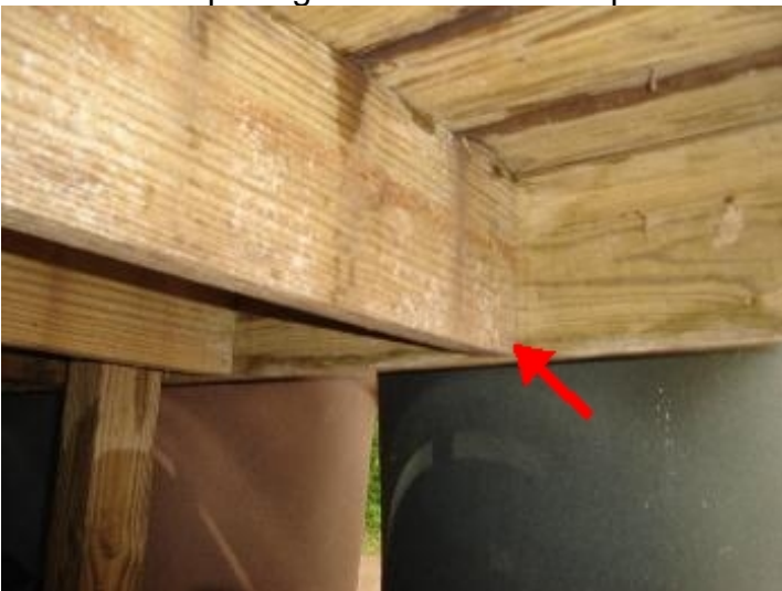
Deck joist installation inadequate. No joist hangers are installed. No ledger board installed.
