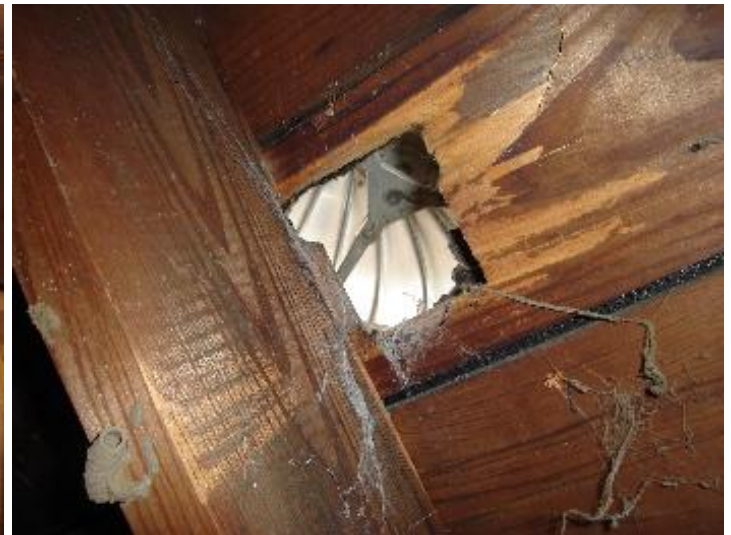
Inadequate opening below roof ventilator. Substantially reduces attic ventilation capacity which is insufficient to start with.
