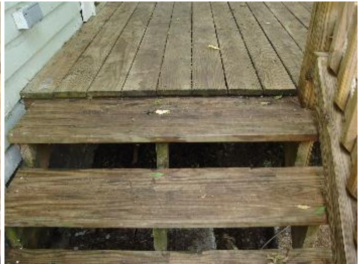
Irregular step riser; potential trip hazard.
