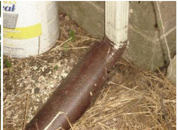
Inadequate downspout diversion potential against foundation. Monitor.
