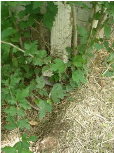
No gutter downspout diversion to remove rainwater away from the foundation.
