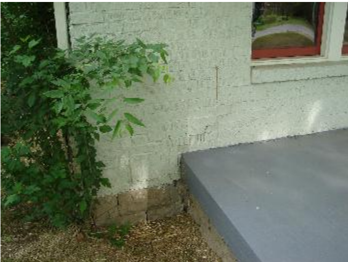
Settling crack with lateral movement. No indication of current activity.
