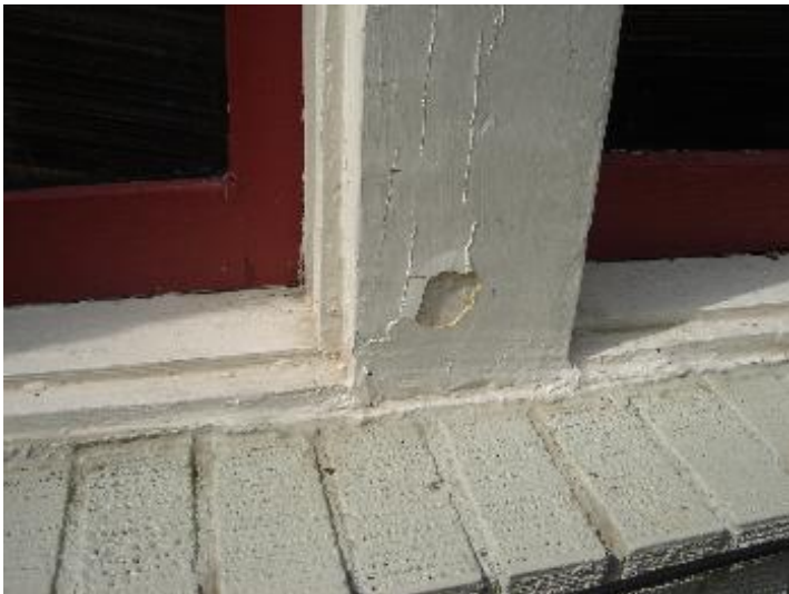
Paint maintenance required. Potential lead paint issue.
