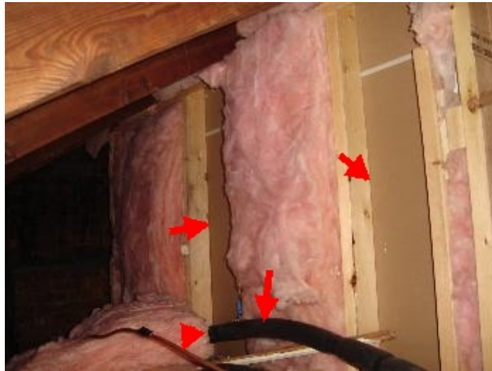
Missing insulation in the bedroom/attic wall. Unsupported refrigeration lines.
