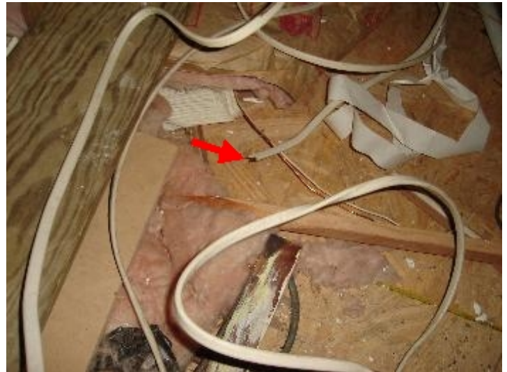
Exposed wiring visible in the attic.
