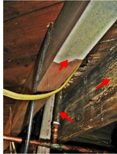
Galvanized pipe still installed on the upgrade copper piping in the house. Staining of the water at the first floor vanity sink was observed above this location.
