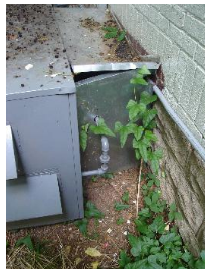
Duct hood openings will allow rodents to enter the crawlspace. May potentially nest in the air duct system and destroy it.
