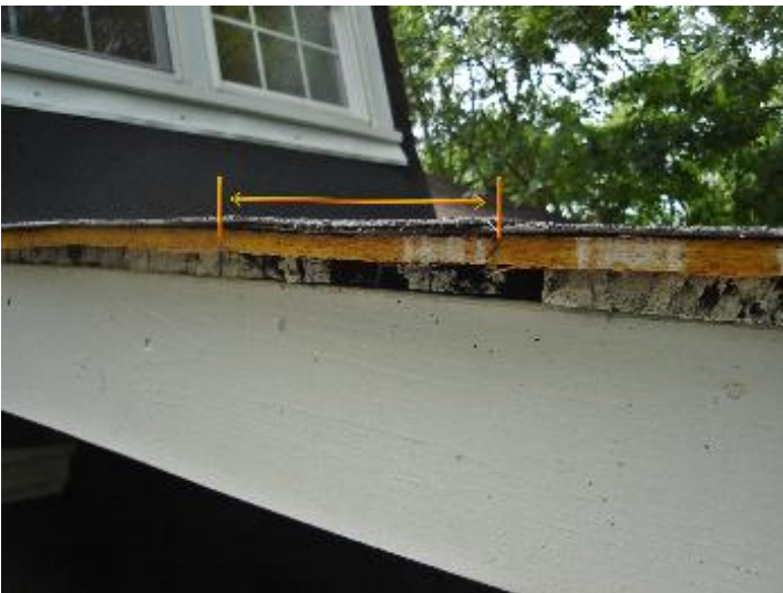
Inadequate overlap of rolled roofing material layers for a low pitched roof. No drip edge flashing installed.
