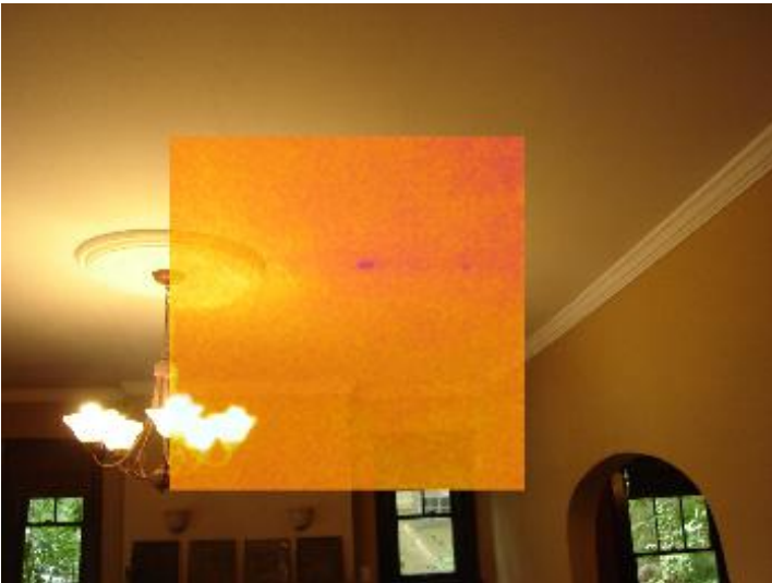
Moisture leakage in the living room ceiling from a leaking HVAC unit above.
