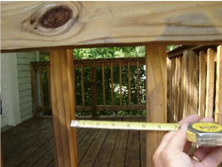
Balusters spacing exceeds 4 inch requirement.
