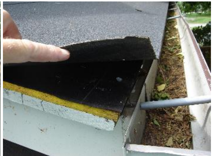
Wind damage at the leading edge of the rolled roofing. Inadequate flashing.
