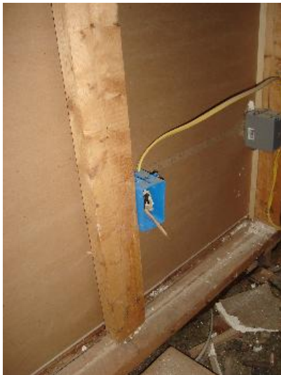
Open Junction boxes. Exposed electrical wiring. Uninsulated interior wall.
