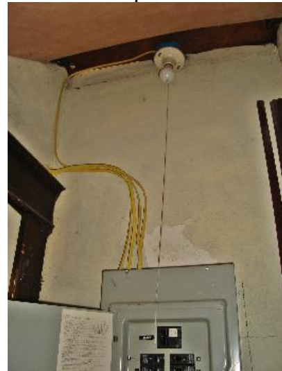
Exposed Romex wiring outside of the finished wall. Improper lighting fixture. Inadequate clearance between in incandescent light fixture any finished wall and ceiling. Light bulb fixtures not protected.
