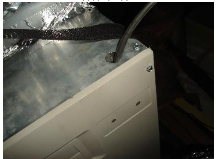
Improper wiring connections at equipment case penetration. Vibration may result in a high voltage ground fault. Interior components of this equipment were not inspected due to safety hazards to the inspector. Wiring may not be appropriately sized. Auxiliary heating banks may not be installed/appropriately sized/have adequate wire capacity/have adequate breakers/fuse protection. Investigate further. The equipment electrical disconnect is attached to the roof decking. This does not conform to industry standards. This panel was not further inspected.
