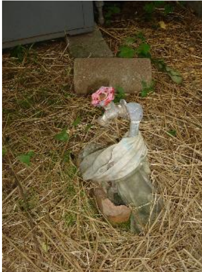
Exterior water supply; no water flow.
