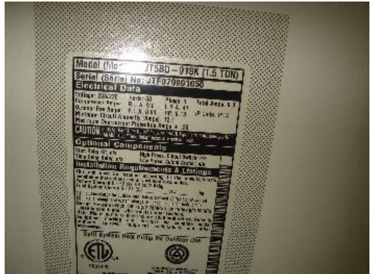
HVAC unit is 1.5 tons for the second floor. There is no indication of cooling load calculation compliance. System may or may not be inadequate for required comfort levels on the second floor.
