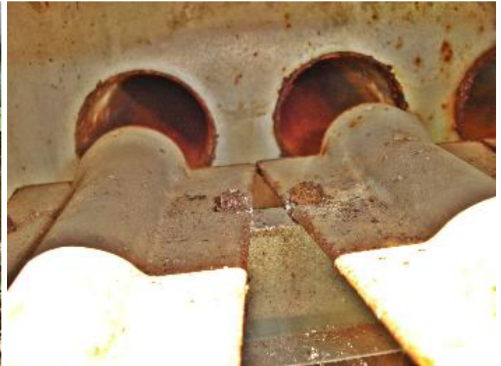
Gas burner/heat exchanger condition. Excessive rusting inside of the exchanger requires maintenance /further inspection by dismantling the unit.
