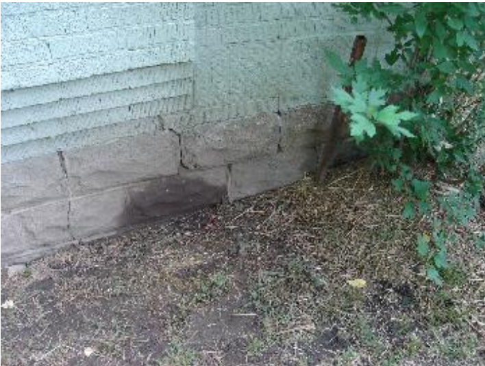
Condensate water on foundation from drain above. Excessive moisture intrusion into the crawlspace. Potential structural damage from expansive soils and hydraulic pressure.
