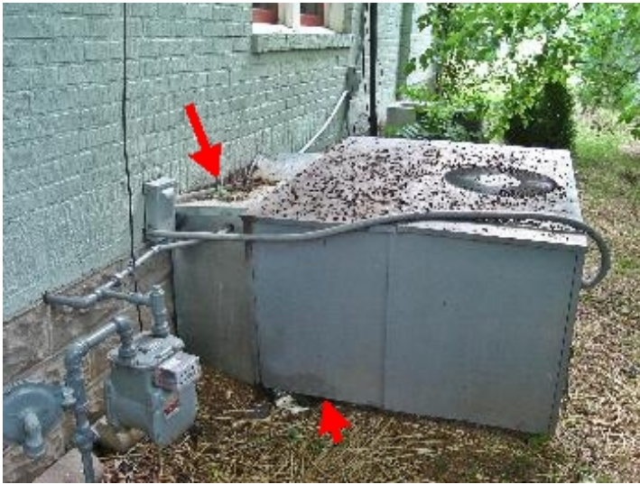
HVAC unit out of level. Condensate flooding the interior of the unit. Indication of freezing evaporator coil. Condensate leaking from service panel. Crushed air duct good between unit and building; source of water intrusion into the crawlspace.
