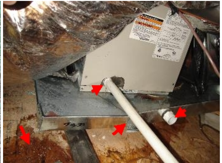
HVAC unit not properly level. Condensate leakage at drain connection. Condensate leakage from flooded interior unit. Auxiliary drain pan cut to facilitate drain. The unit should be raised above this level. Condensate leak out the pan. Condensate drain pan is not level. Condensate drain pan overflow piping not installed. Condensate drain does not have a trap installed as required (this will cause the coil pan to overflow during operation; it is also an efficiency concern as unconditioned outdoor air will be drawn in through the pipe.). Obvious water leakage on the attic flooring (resulting in ceiling damage below). No drain pan safety switch installed to shut down the unit in the event of an overflowing pan due to a condensate leak.
