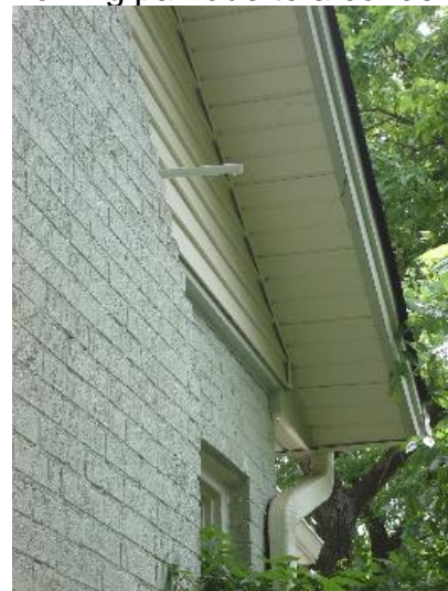
Improper condensate drain line termination from HVAC equipment.
