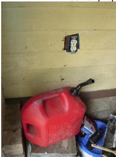
Exposed electrical outlet.
