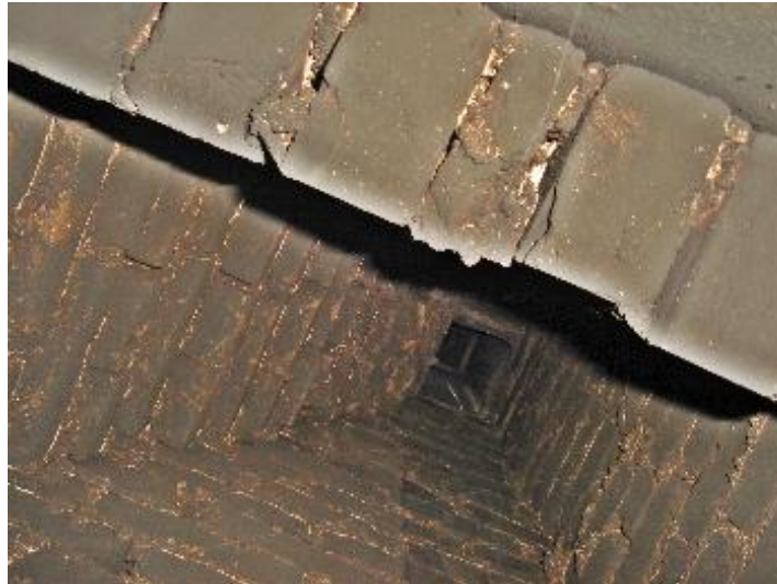
No flue damper in the fireplace. Efficiency concern.
