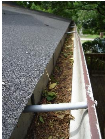
Gutters clogged with tree debris. Improper nailing of the rolled roofing.
