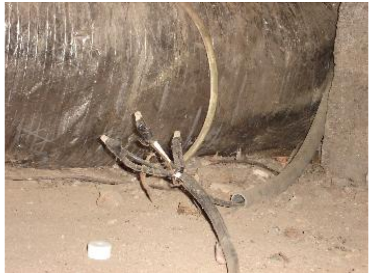
Exposed high amperage wiring to the HVAC equipment; not installed in an approved junction box or properly attached to the house framing.
