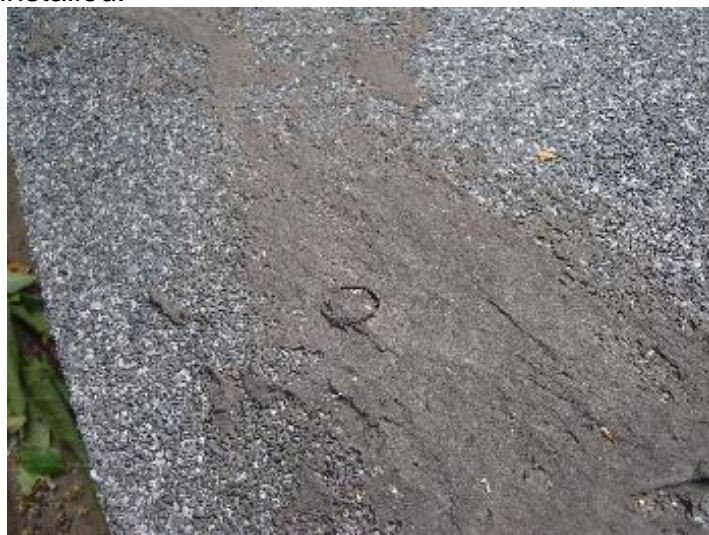
Deterioration of roofing cement at nail heads. Potential water damage to the sub-roofing.
