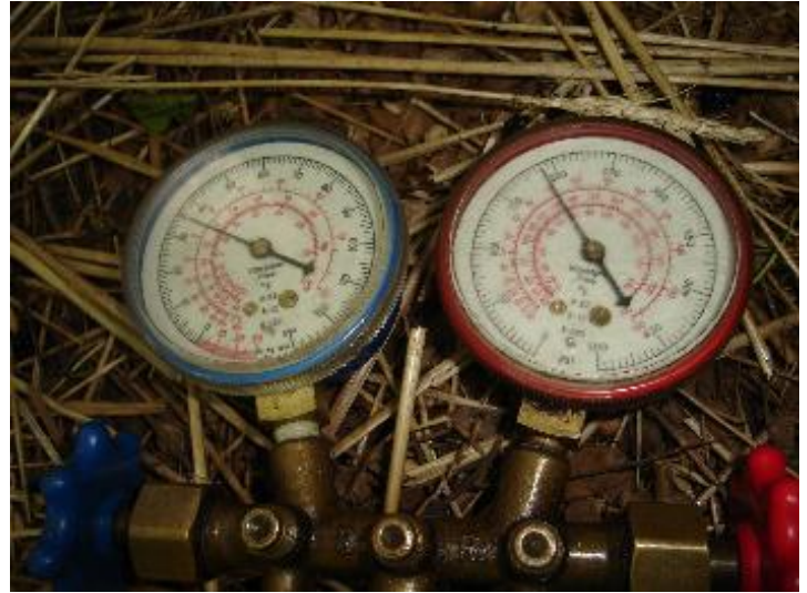
Low refrigeration pressures. First floor unit.
