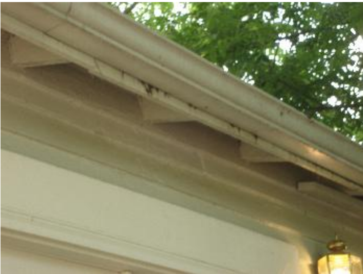
Indication of back flowing gutter; tree debris.
