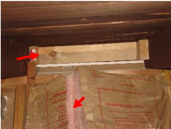
Roof Rafter ventilation is sealed above the knee wall. Baffles are required for adequate ventilation of the roofing system. This also increases heat gain on the cooling system.
