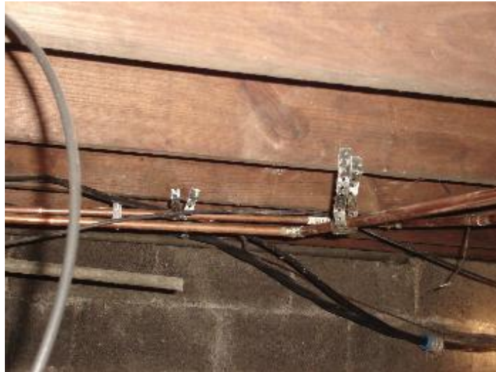
Improperly supported plumbing lines. Improper fasteners and inadequate support schedule.
