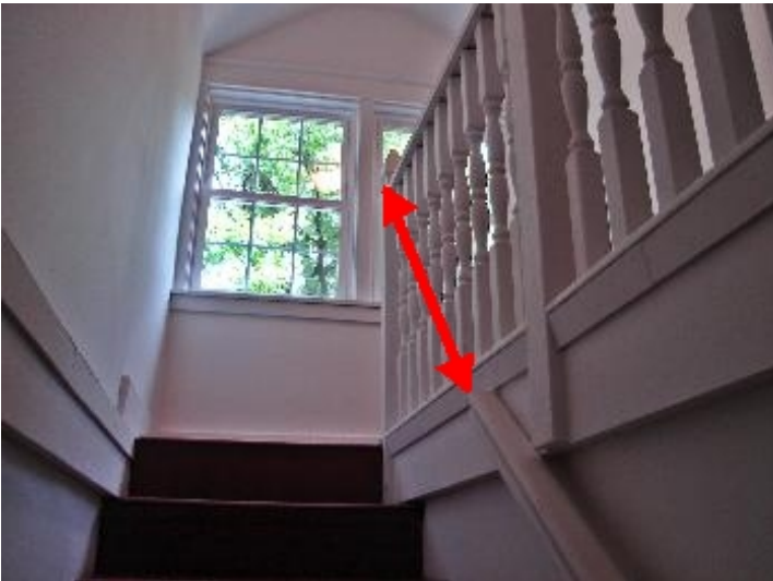
No handrail at the top risers of the second-floor stair system.
