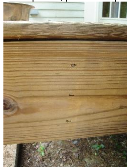
Joists are end nailed with three small pneumatic nails. Deck failure potential under load. Joist hanger installation required.
