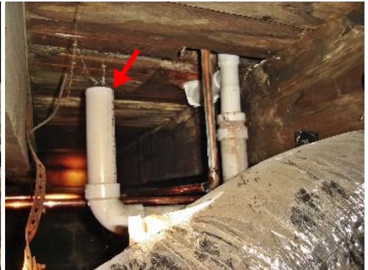
Waste drain is open to the basement atmosphere. No pipe cap installed.
