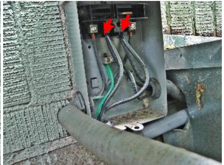
Double tapped HVAC disconnect panel. Electrical wiring overheated. No fuse protection for wiring/HVAC equipment on either HVAC subpanel.
