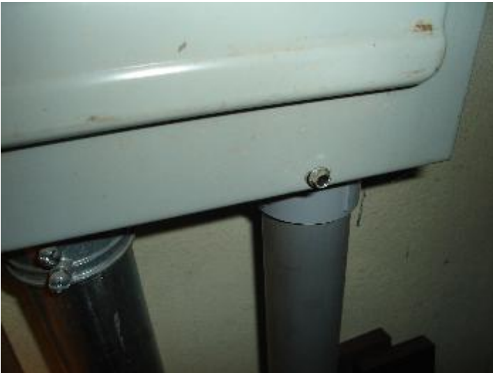
Sheet metal screws utilized on electric subpanel cover. Main electric subpanel was not inspected due to this hazardous condition.
