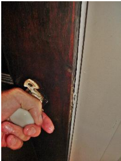
First floor bathroom entry door does not close, latch, or secure. Privacy is expected at bathroom locations.
